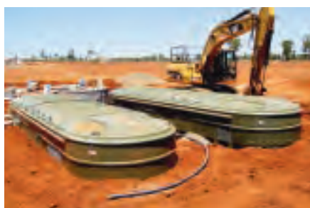
Large BioDisc wastewater treatment systems - Mining Project, Queensland Australia
